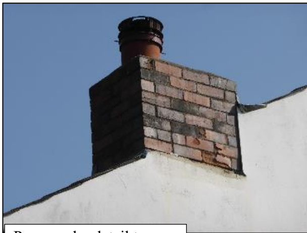
Poor render detail to South West chimney CH01
